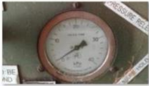
Roof Tile TBS 001 Hydraulic Pressure Gauge at approx 1.8MPa (Max deflection)
