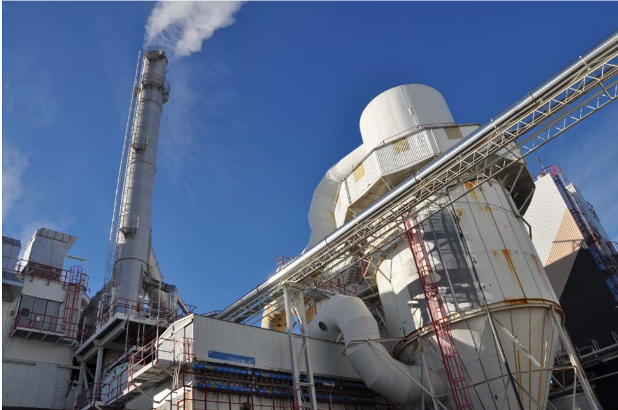
PVC plant, Sweden
