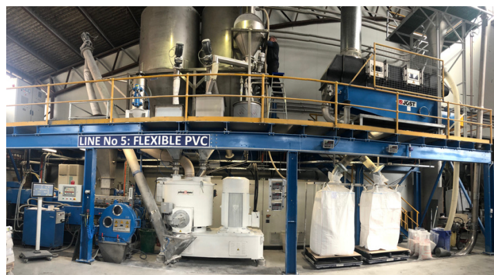
The PVC manufacturing plant at RBM Plastic Extrusions
